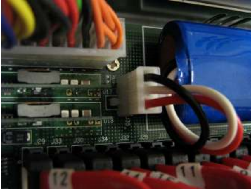
Figure D-4 Battery Plug Locked in Place
