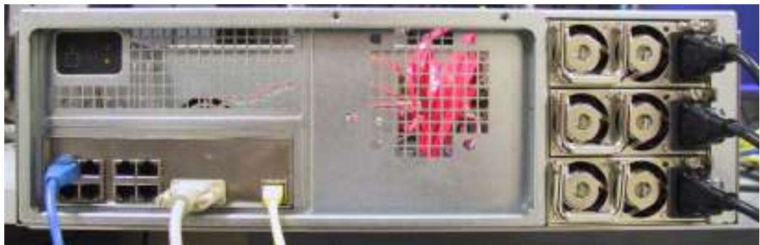
Figure F- 2 Rear View of Enclosure
